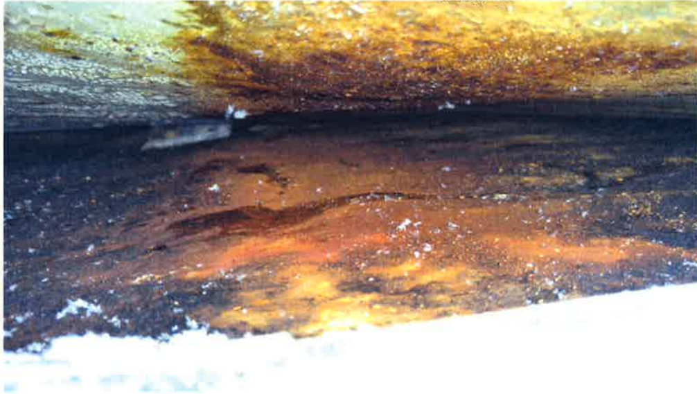
Photograph 3: Corrosion present on the underside of the metal roofing
