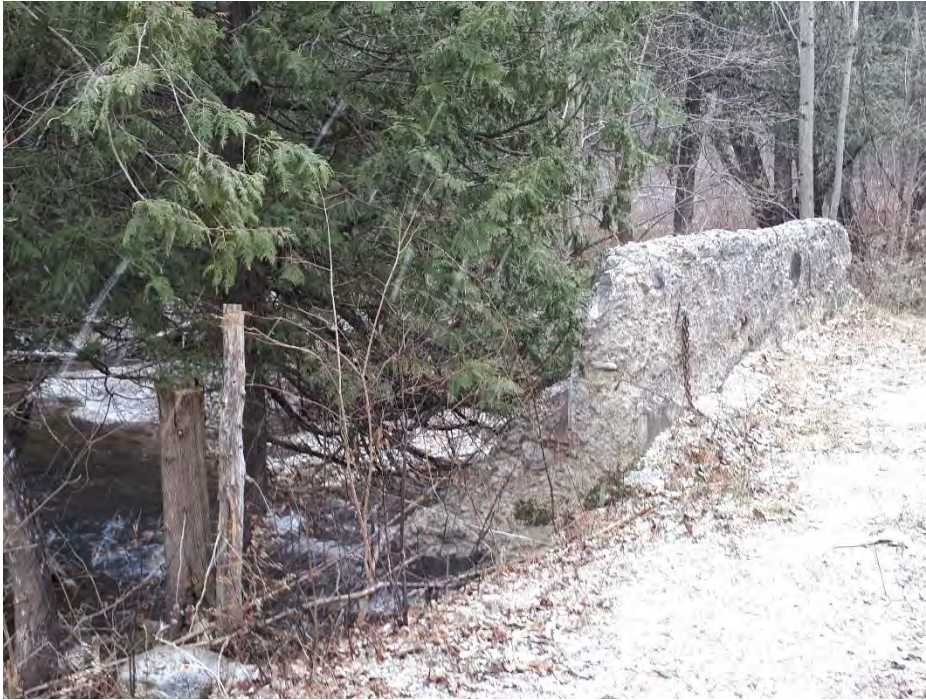
Image 19: Unmarked old Stone and concrete bridge crossing the Pretty River, facing south-southwest.
