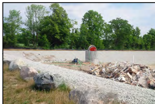
LEACHATE COLLECTION CHAMBER
