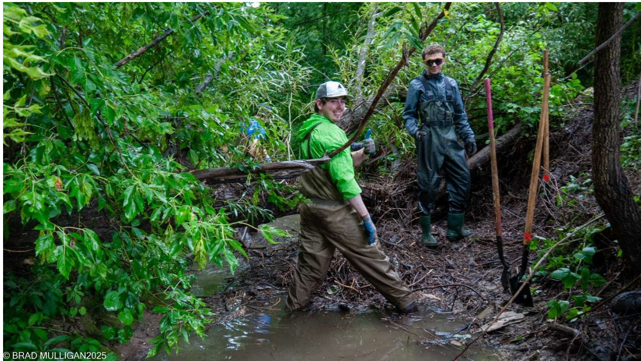
Example of Blockage before
